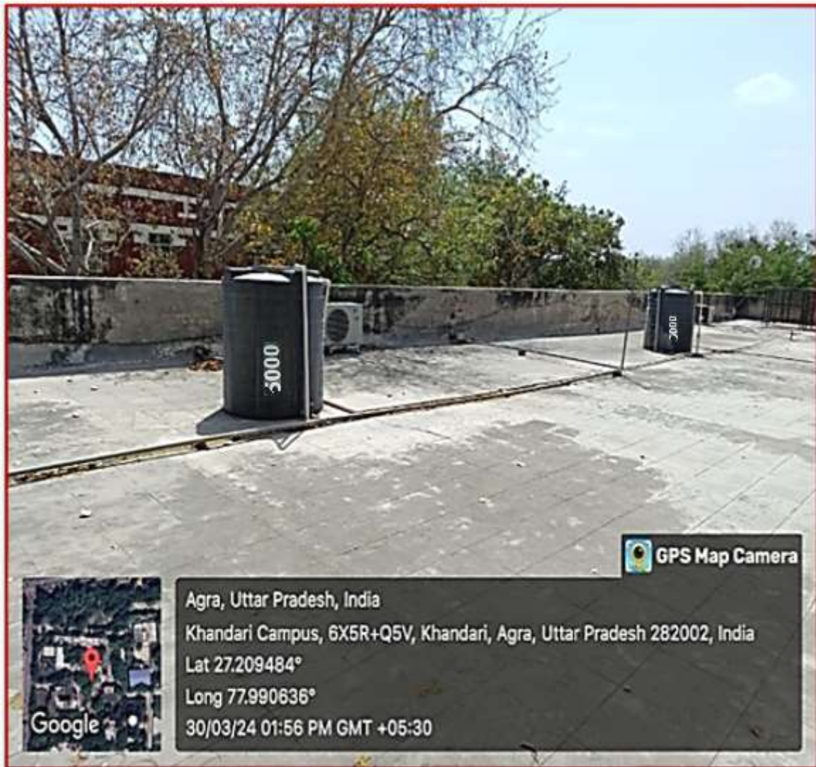
Water distribution Tanks
