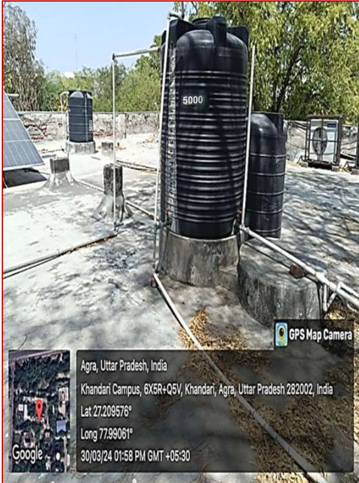
Water distribution Tanks
