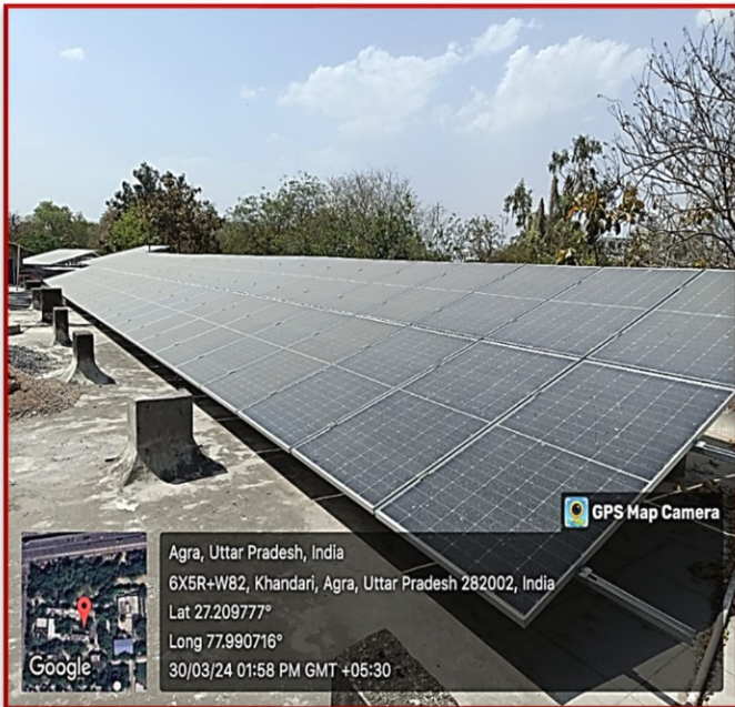
Solar Power System University Campus – 60KWh
