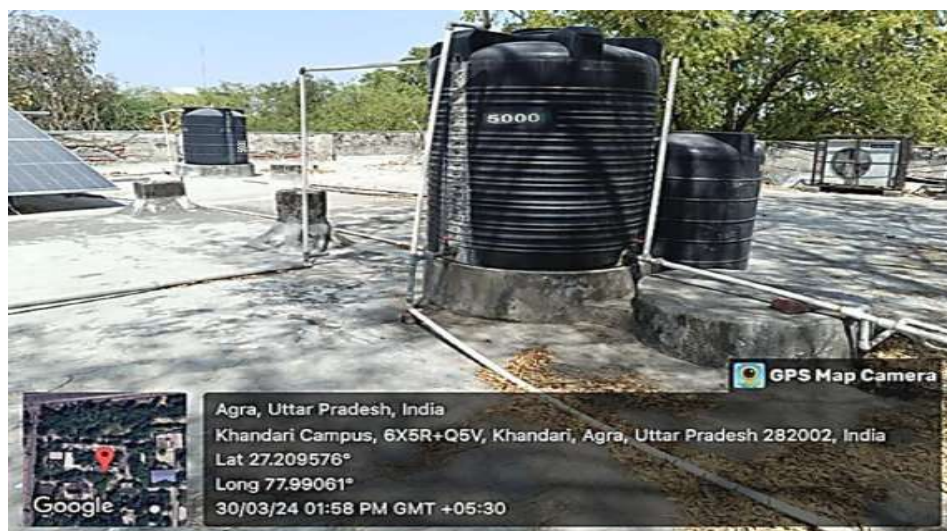
Water distribution Tanks
